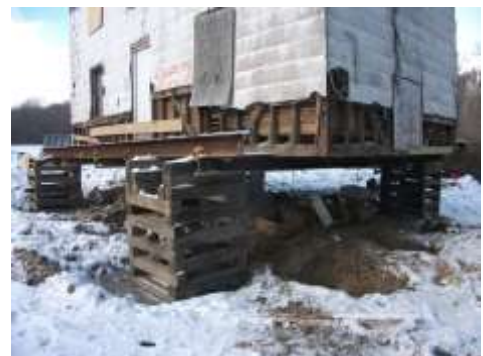
Above: Stabilization of the structure involved lifting it to repair the framing and replace the foundation.
