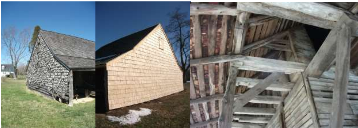
Above left and center: The corn crib's shingles before and after restoration.
